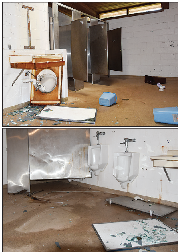
The vandalized bathrooms at Tourist Park
