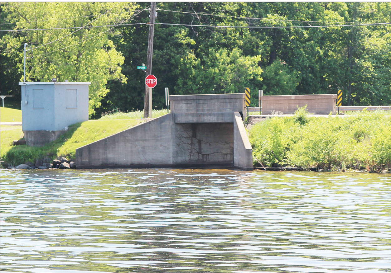
The culvert at the heart of the issue. The complete DOT Study, with drawings, is available for reading at City Hall.
