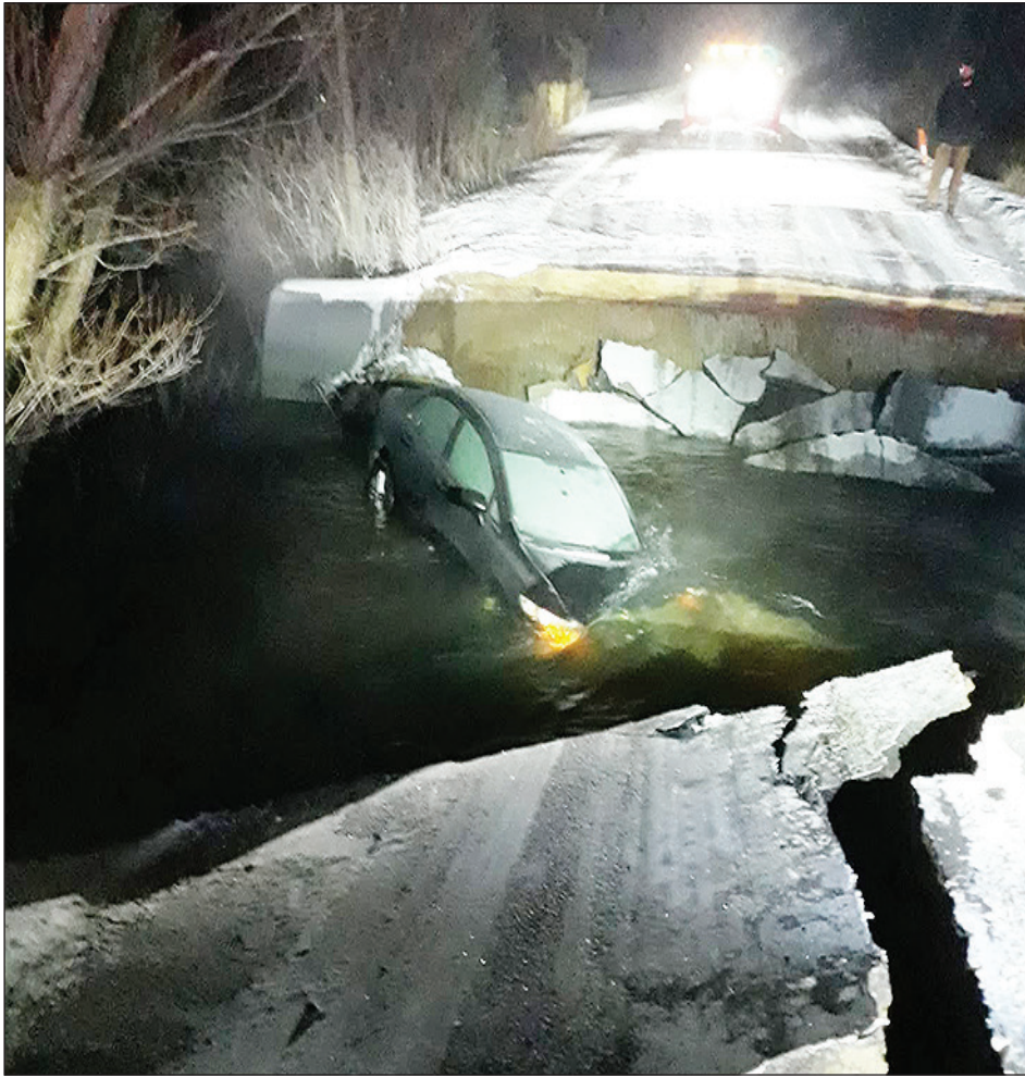
Authorities in Northern Wisconsin are warning residents about a wash out between two lakes and how part of the ice and snowmobile trail is not safe. According to the Washburn County Sheriff’s Office, on February 2nd, a culvert between Little Mud Lake and Long Lake failed. Officials say the washout is around 40 to 50 feet wide and is not passable.
