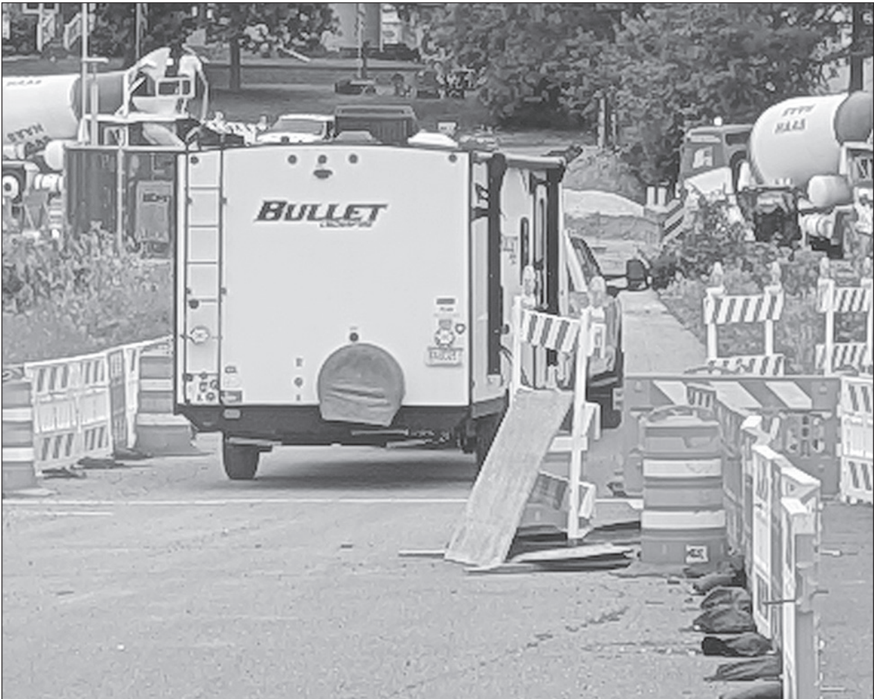
Even with all the barricades and signs, some drivers still try to make it through the Highway 63 bridge closure. This truck and camper made it part way and were forced to back out. You can't make it up!
