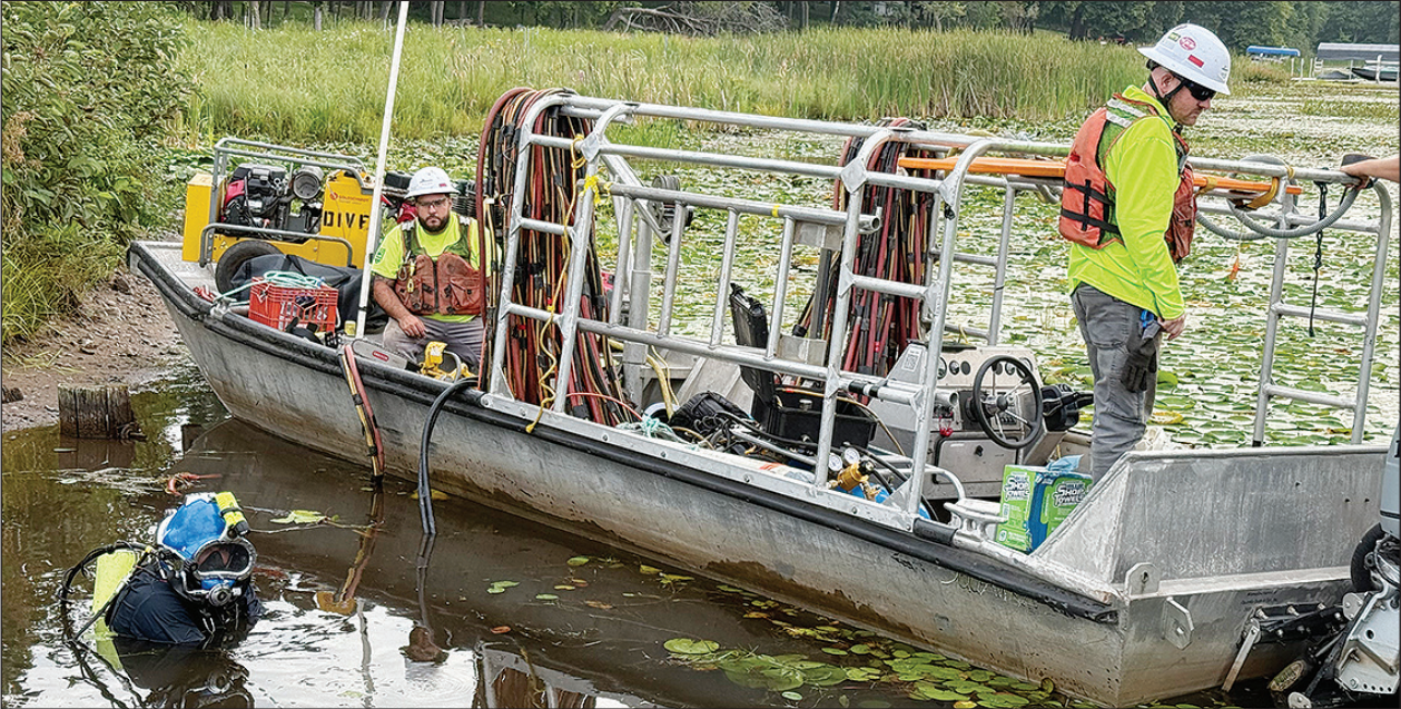
Trestle Obstructions (July 8, 2026)
